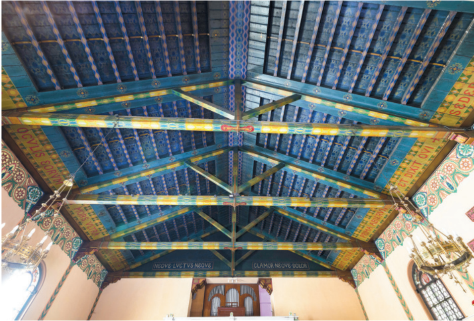
Fig. 12. Church of the Resurrection of the Lord in Cracow. Interior, roof truss with polychromy from 1886, designed by Father. L. Zbyszewski CR, made by Karol Orlecki's firm.
