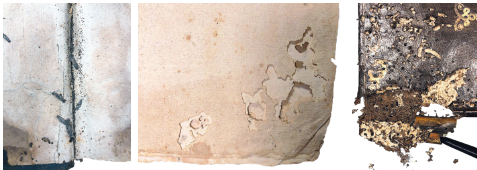
Fig. 4-6. Paper loss and cover damage alongside leather binding due to long-term insect infestation. Document from the Archives of the Resurrectionist Fathers in Rome.
